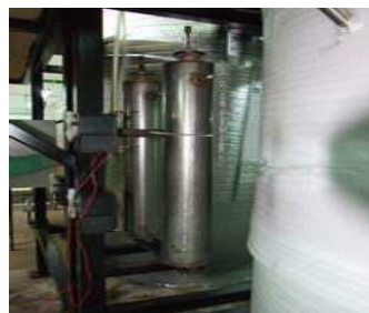
Figure 10 – the H 2 S filter (in the back) and the CO 2 filter(in the front plan) of the installation. Also in front of the two filters there are the pumps that will be commanded by the pH sensors of the installation.
