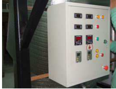
Figure 11 – The electric panel of the installation
