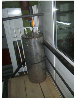
Figure 12 – The biogas storage tank
