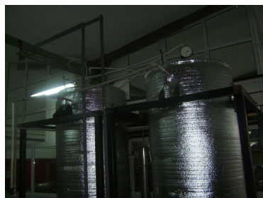
Figure 9 – Front view of the biogas production installation
